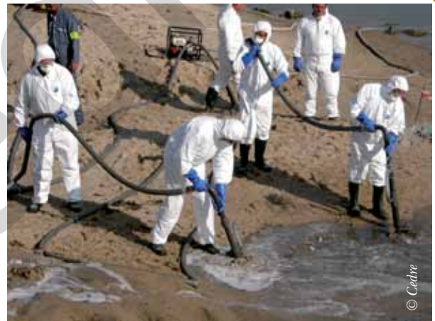
Flushing enables highly selective recovery of buried pollutant without taking too much sediment
