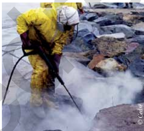
Risks of pollutant splashing
